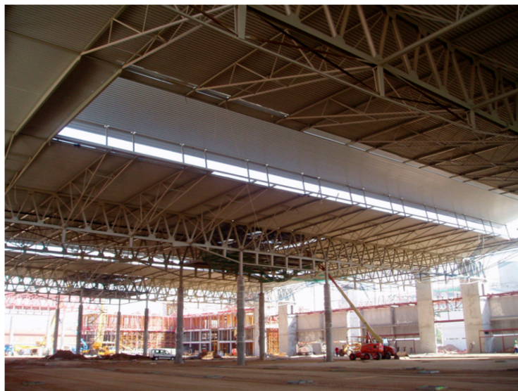
Figure 14. View of the nearly completed two-module steel structure. Photograph by the author.
