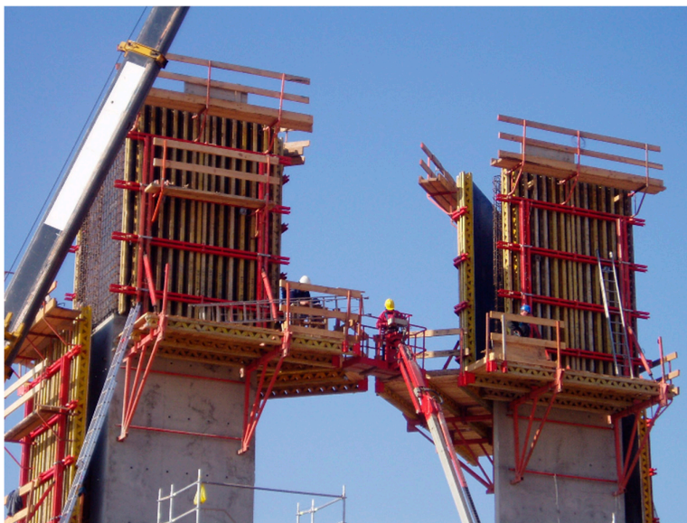
Figure 13. Formwork closure process prior to concrete pouring. Due to the scale of the project, the entire operation had to be carried out using mobile cranes. Photograph by the author.
