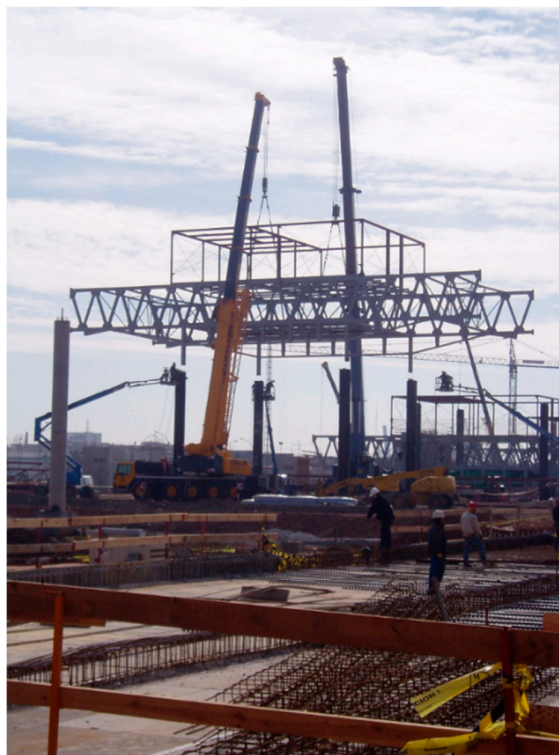
Figure 12. Lifting of the central core of a typical module. The image shows two cranes performing the lift, and four mobile cranes, with four operators, securing each of the legs to the concrete pillars. In the background, a second module awaits lifting half an hour later. Up to five modules could be lifted in a single morning, optimizing the performance of the mobile cranes. Photograph by the author.
