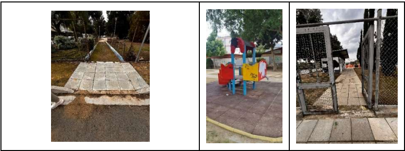
Figure 18. Zone G- Neglected Section-b.
