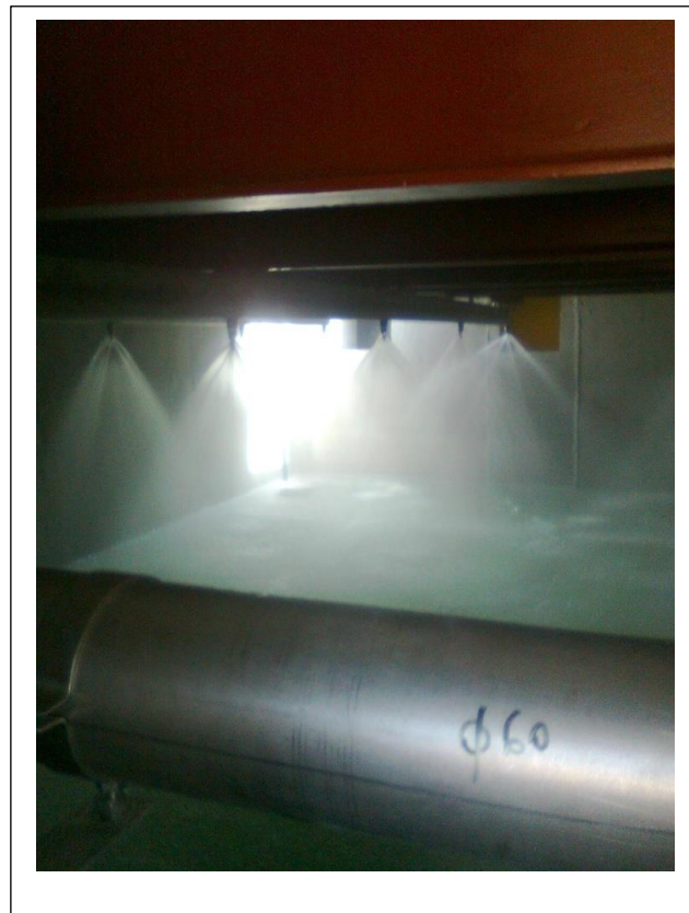
Figure 3. Illustrates the membrane rejectors, which maintain a residual pressure of approximately 1 bar. This pressure is utilized to spray the contents back into the bioreactor, facilitating oxygenation.
