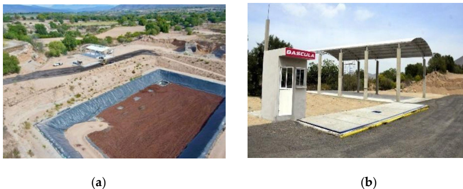
Figure 5. (a) The SAIRSUME construction, aerial view; (b) The SAIRSUME infrastructure for weighing and waste classification.
