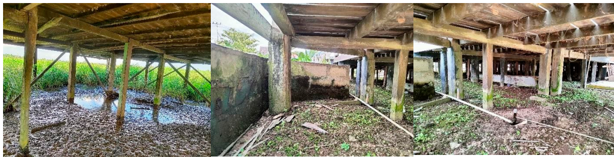
Figure 8. Foundation Condition with Dry Areas
