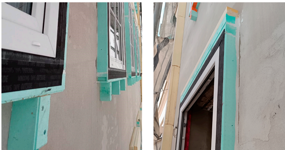
Figure 4. Window installation within the insulation layer using a load-bearing thermal insulation profile – example from a construction site.
