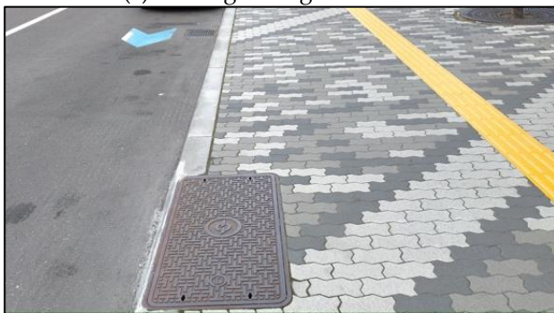
(e) Closed Manhole located on edge
