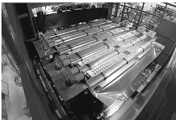
Figure 17. Photograph of the collector plate situated at the rear of the explosion-proof chamber. A total of 480 high-voltage coaxial power cables (30 m in length) from the capacitor modules, located in the adjacent room, are connected to the collector plate from the bottom. [Photograph taken by the author at ISSP, The University of Tokyo.]
