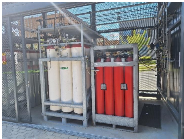
Figure 14. Hydrogen storage tanks installed in the gasification facility
