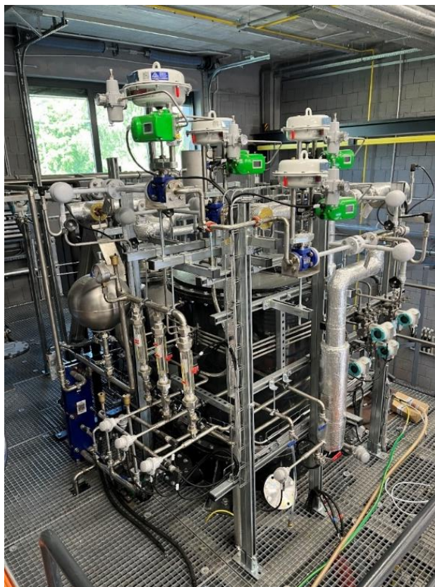
Figure 4. Gasification facility with the reactor at the core of the process.
