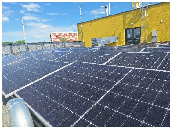
Figure 18. Photovoltaic and wind energy systems installed in the facility
