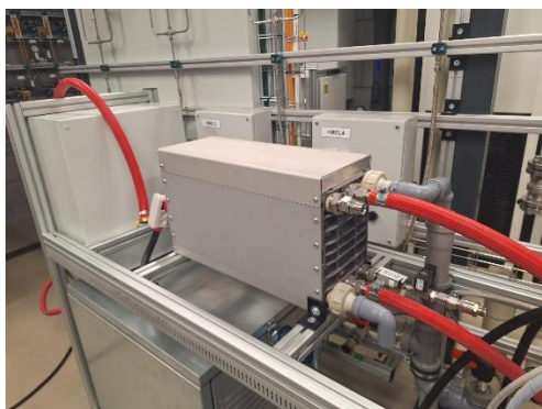
Figure 15. Installed Nedstack FCS 8-XXL fuel cell stacks as part of the system for hydrogen-to-electricity conversion
