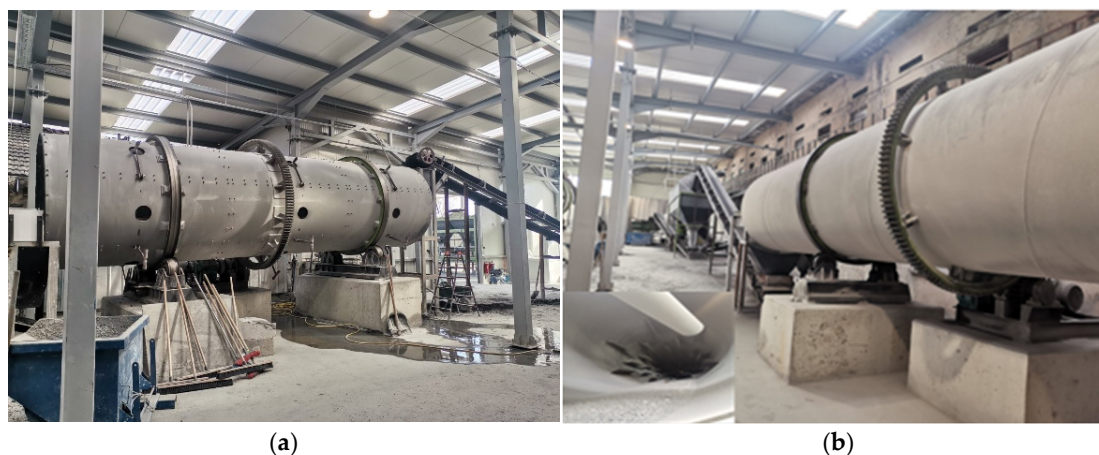
Figure 3. Delivered and constructed facilities by Green circle biotech Ltd. at the Polski Trambesh site: (a) Drum granulator; (b) Heater.
