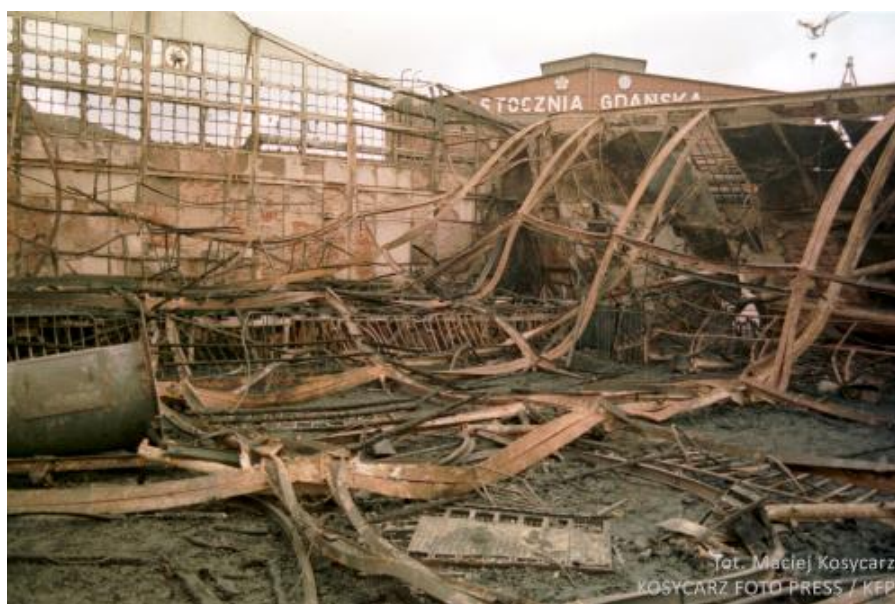
Figure 6. Burnt hall viewed from the inside (Maciej Kosycarz/KFP).
