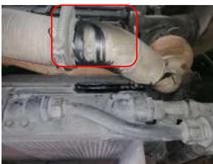
Figure 10. Engine oil leak.
