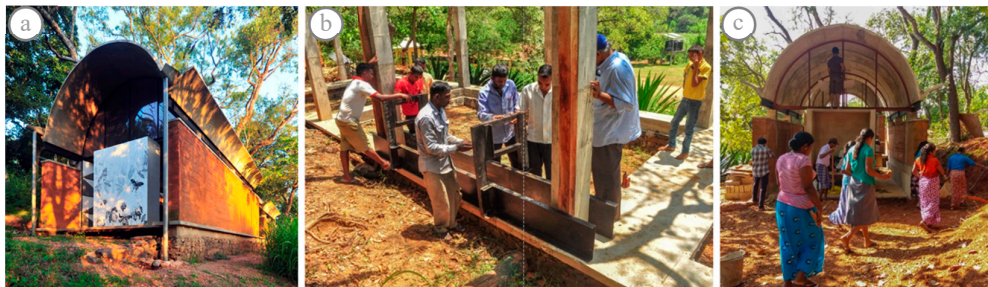
Figure 2. (a) Dewahuwa school learning pods; (b-c) the parents, volunteers and village builders supporting the construction activity.
