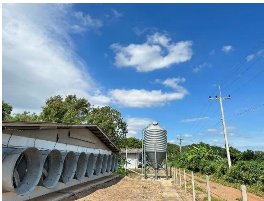
Figure 4. Application for ventilation fans.
