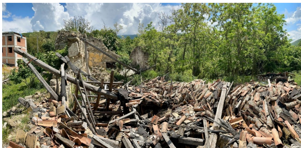
Figure 1. Heterogeneity of materials in a building that collapsed following the 2016 earthquake in Central Italy, Accumoli (RI).
