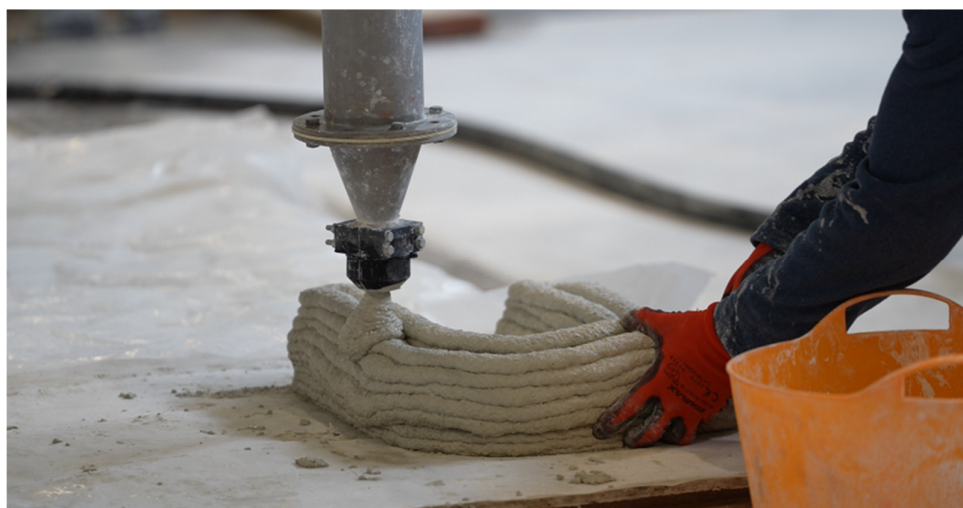
Figure 5. Failed 3D concrete printing.
