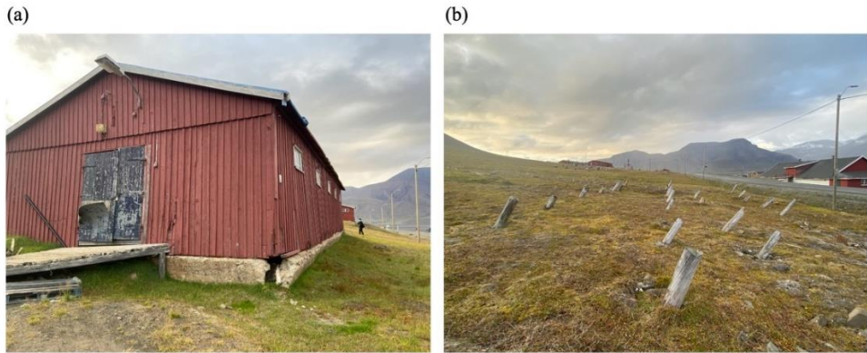
Figure 2. The impact of the thawing permafrost on construction in Svalbard. (a) Warehouse damaged and (b) Slanted house foundation due to permafrost thawing.
