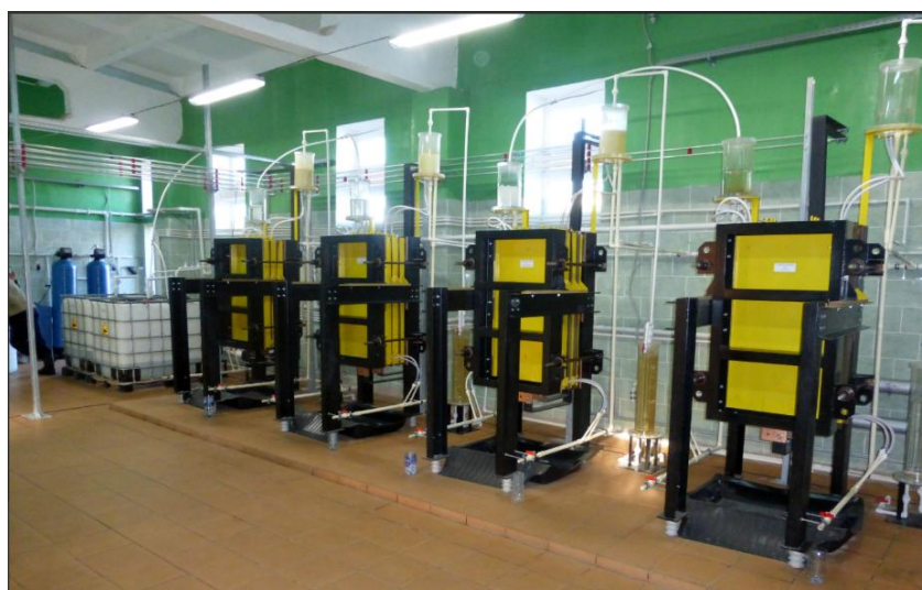
Figure 3. Appearance of an Electrochemical Wastewater Treatment and Separation System for Industrial Use.
