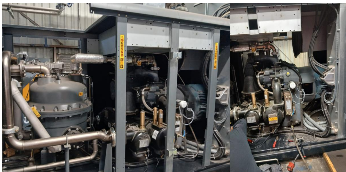
Figure 14. Picture of the compressor N°4 with all components during the annual maintenance.
