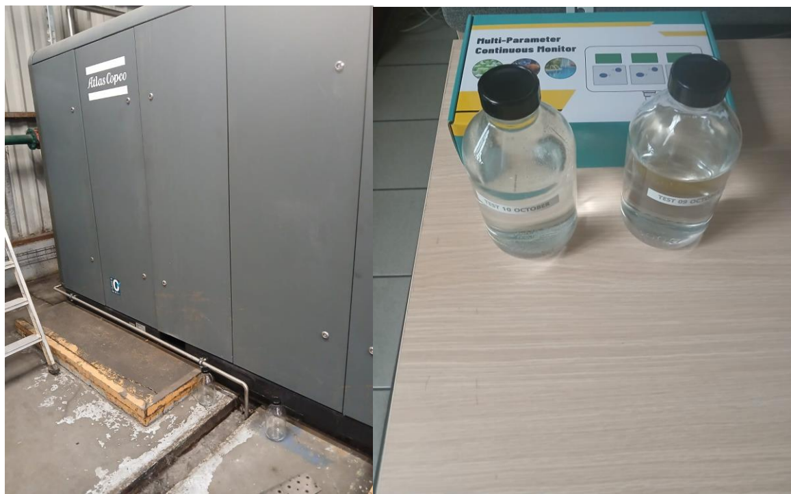
Figure 16. Picture of the compressor N°4's condensate drain and the two bottles used for separate field measurements on October 9th and 10th.
