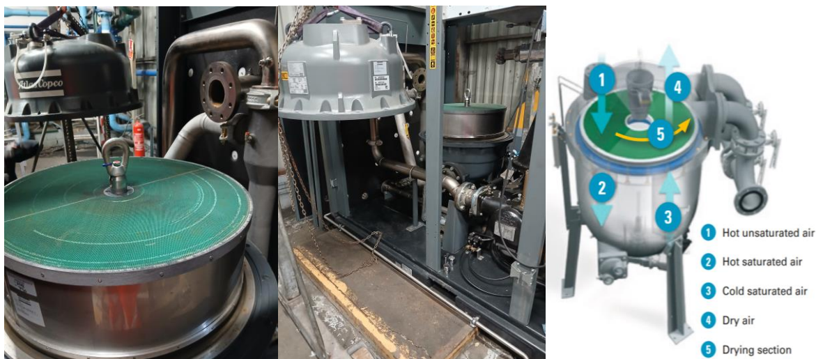
Figure 13. Picture and schematic of the rotary drum dryer (N°10 in Figure 12) of compressor N° 4 during the annual maintenance in August 2025.
