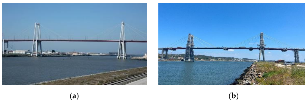
Figure 3. Photograph of the Edgar Cardoso Bridge: (a) before rehabilitation; (b) under rehabilitation.
