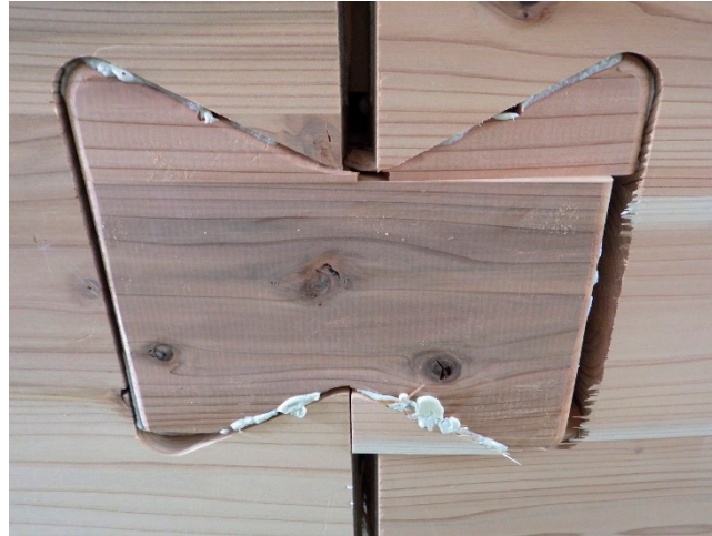
Weak axial crack with shear key
