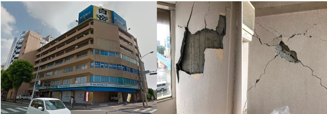
Figure 9. Shear-Failure Cracks in a Reinforced-Concrete Shear Wall (Authors).
