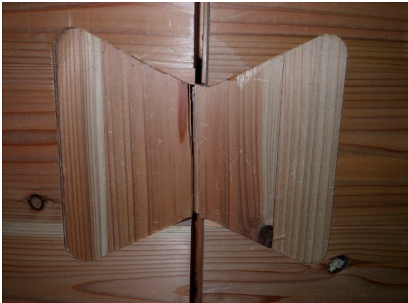
Crack fracture along fiber direction
