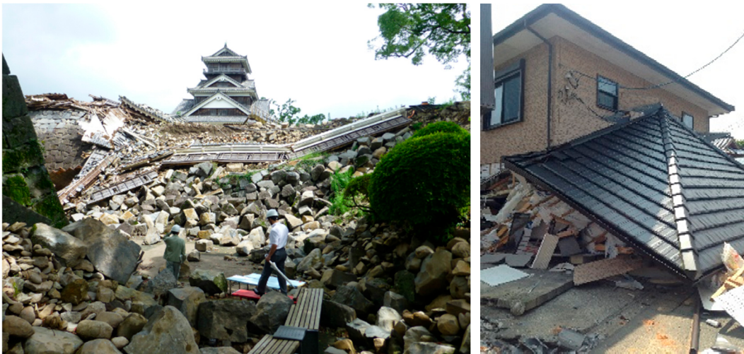
Figure 1. Consecutive Kumamoto earthquake damage (Authors).
