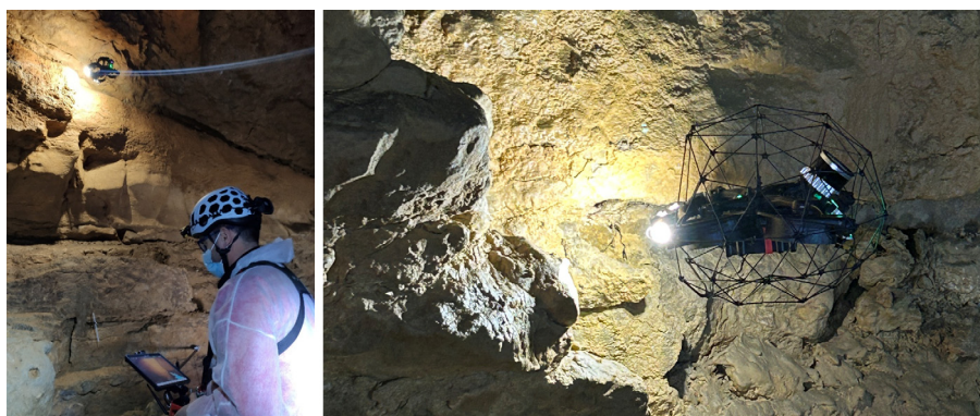
Figure 6. Data acquisition and inspection process with the confined-space UAV, using LiDAR-SLAM navigation and simultaneous video capture for videogrammetry.
