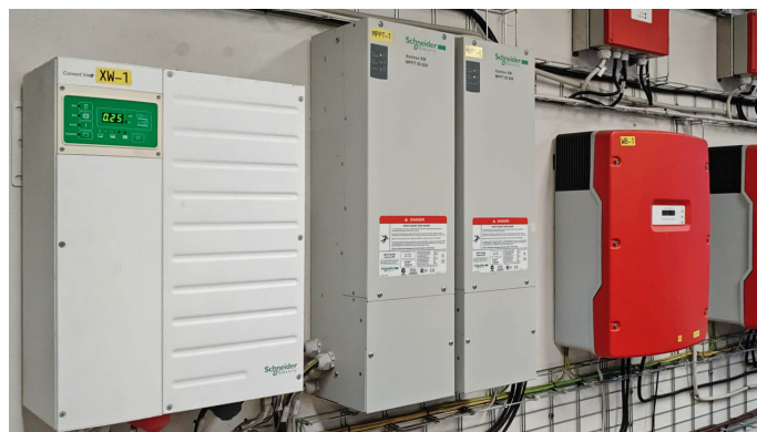
Figure 4. Hybrid inverter Conext XW+ 8548 and PV inverters Xantrex XW 80 600
