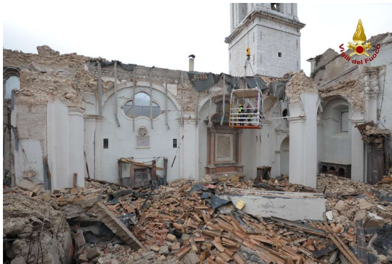
Figure 2. Co-cathedral of Santa Maria Argentea in Norcia during the safety and rescue operations carried out by the Firefighters on November 12 nd 2016, a few days after the earthquake. (Credits: Vigili del Fuoco; https://www.vigilfuoco.tv/umbria/perugia/norcia/recupero-opere-religiose ).
