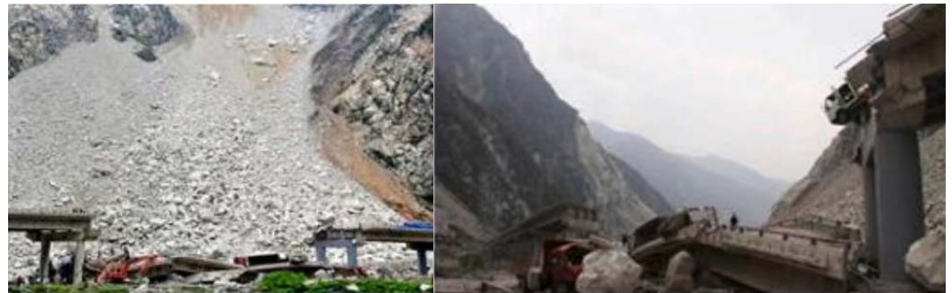
Figure 1. Bridges impacted by rockfalls.
