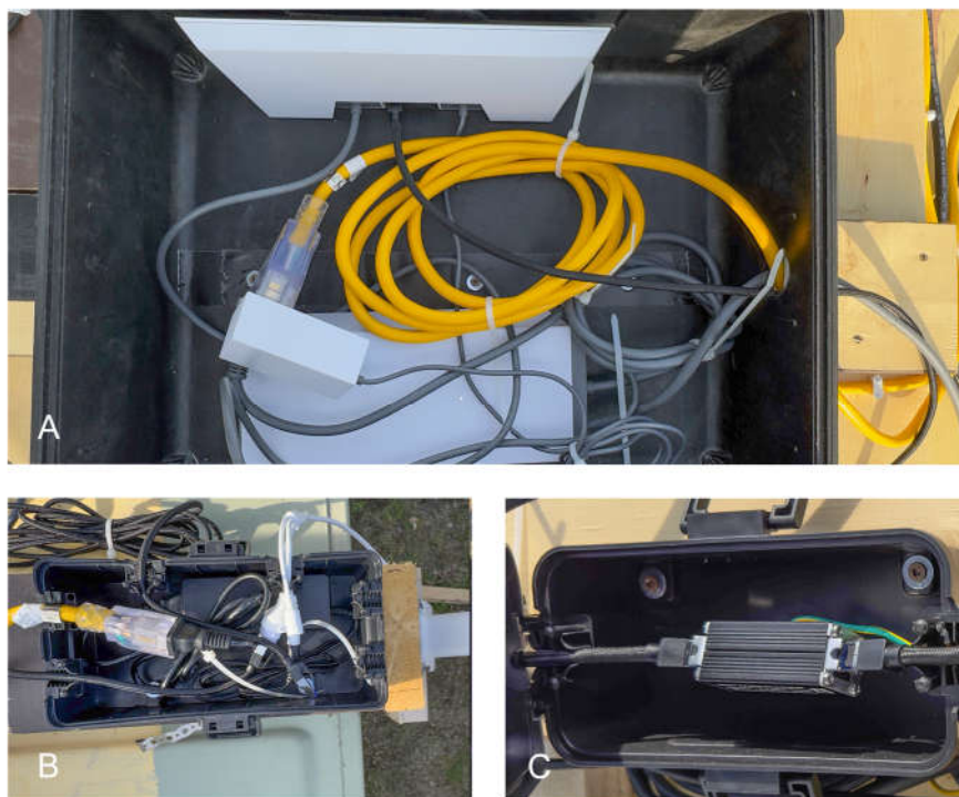
Figure 3. Interior view of A) Pelican case housing the Starlink modem and power supply (Figure 2:H), B) Waterproof electrical box housing the power supply and Ethernet connection for the security camera, C) Waterproof electrical box housing the RJ45 surge protector (Figure 2:J). The bundled but unplugged Ethernet cable shown in (B) was used during on-site testing and setup of the Dock 2 to connect a laptop directly to the
