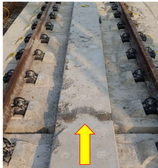
Figure 16. Damage status of DCP after collision.
