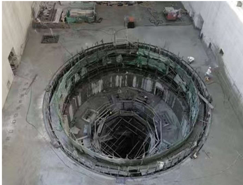
Figure 2.7. Zambian hydroelectric project.
