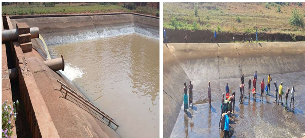
Figure 4. Storage reservoir at Nasho GFI scheme.
