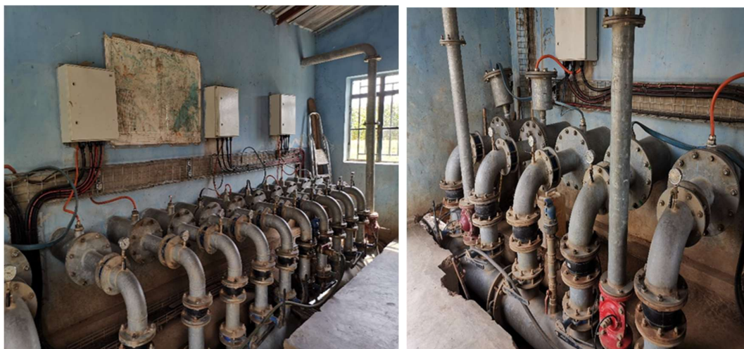
Figure 8. Conveyance pipeline Kagitumba irrigation scheme.
