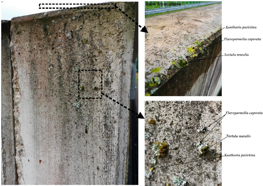
Figure 3. The signs of the third stage of biological colonization on a 9-year-old concrete wall: growth of lichens and mosses starts at the corners, cracks, and surface irregularities.
