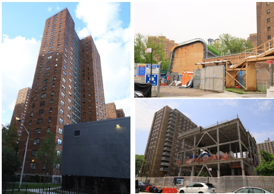
Figure 3. Restoration works as part of Sandy Recovery Program at several public housing developments in NYC.
