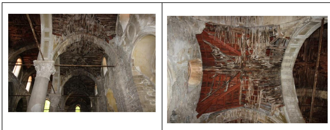
Figure 8. Damages and Material Losses in the Roof System (Author's Personal Archive).
