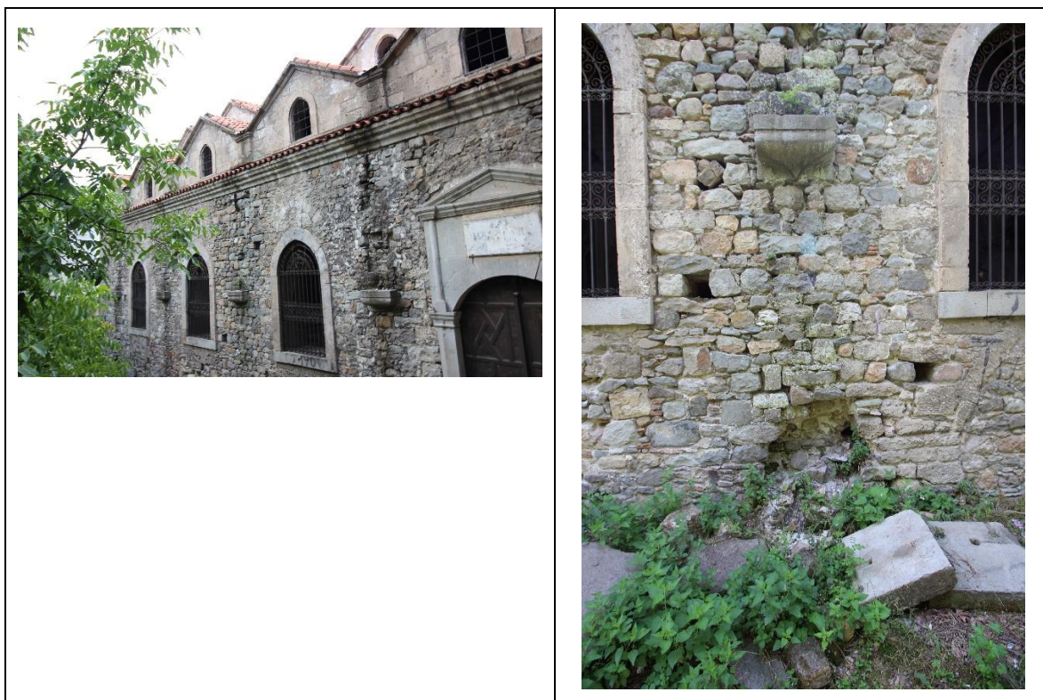
Figure 9. Moss and Lichen Colonization with Surface Degradation on the Northern Elevation (Author's Personal Archive).
