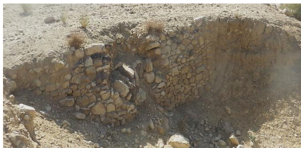
Figure 1. Collapsed terrace wall with intact fill.
