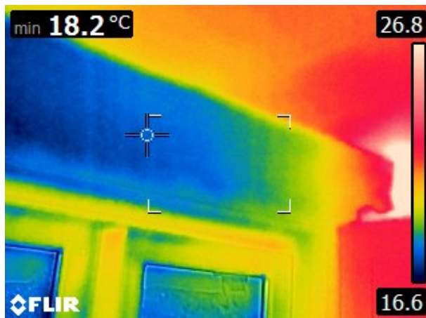
Image 1. Cold External Wall Surface – TUD004 Kitchen.
