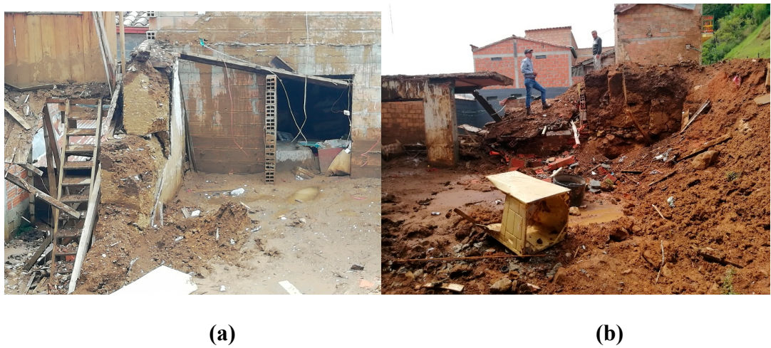
Figure 13. (a) Affected building 1 st Avenue – 7 th Street, left side. House 6. Earth wall detail; (b) Affected building detail 1 st Avenue – 7 th Street, left side. house 6.
