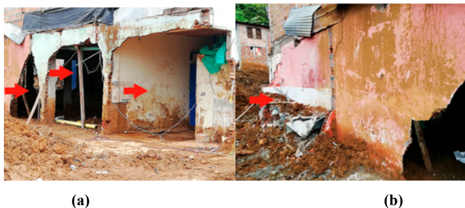
Figure 6. (a) Side facade, infill walls total collapse, House 2; (b) Side facade. Infill walls without total collapse. House 2.
