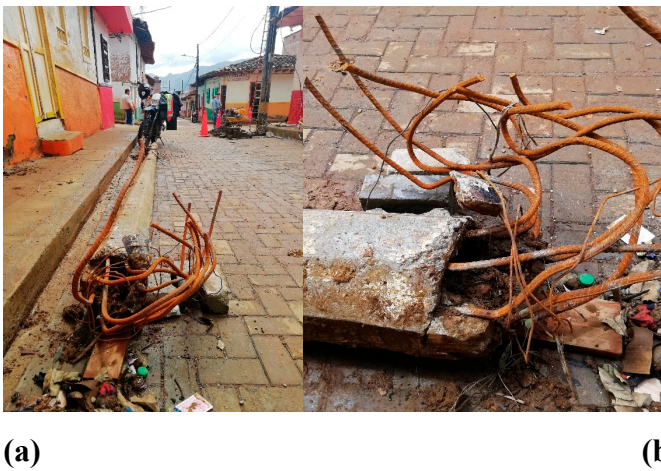
Figure 14. (a) A power pole collapsed on 6 th Street, lower slope of las Nubes Hill; (b) Collapsed power pole on 6 th Street, lower slope of las Nubes Hill.
