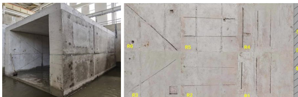
Figure 3. Schematic diagram of the construction layout of the test platform and the cracked wall.
