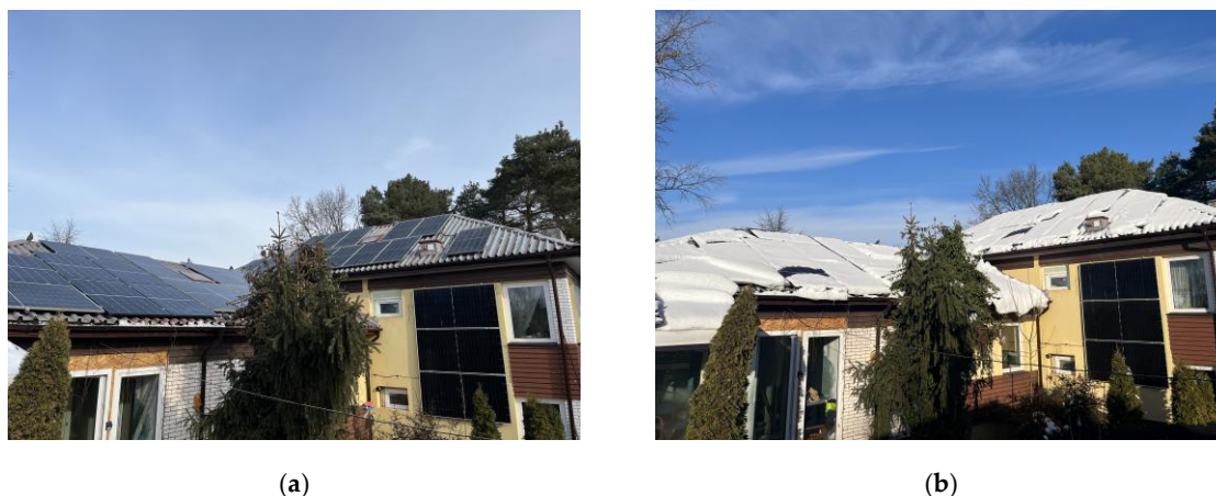
Figure 3. Case 2 balcony PV installation – detached building with roof-top and facade PV, comparison of panel operating conditions during: (a) autumn; (b) winter, where the roof panels are almost completely covered with snow, while the vertical panels on the façade remain exposed to sunlight and produce energy [Own source].
