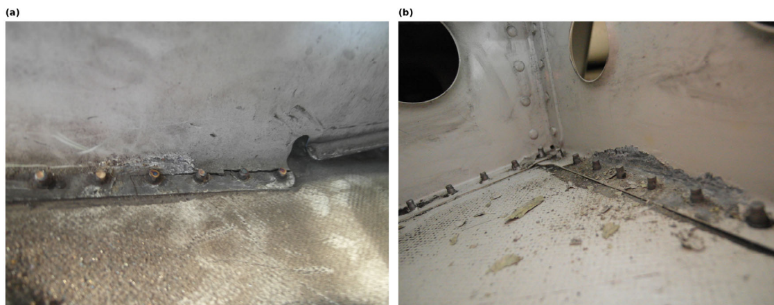
Figure 6. Field inspection evidence of corrosion in a hidden aircraft zone after prolonged persistence of corrosion-prone conditions. (a) Close-up view of corrosion damage developing along a riveted and lap-joint-type detail. (b) Wider view of corrosion products and degradation in a hidden structural zone. These findings
