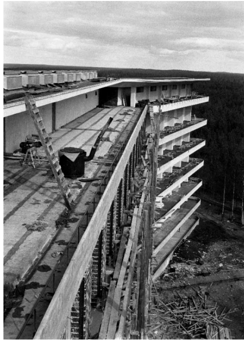
Figure 1. The patient wing building site in autumn 1930. The A-wing pillars on the external wall line were cast in situ and protected by a bricklayer. Photographer Alvar Aalto or Aino Marsio-Aalto. Photo No. 50-003-079. AAM.
