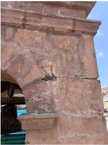
Figure 6. Visible cracking and surface deterioration in the tower, consistent with its reduced effective stiffness.
