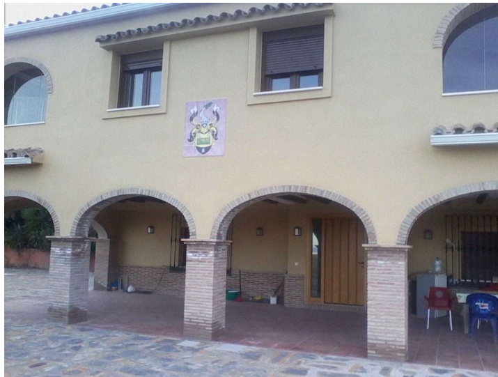
Figure 11. Current state of the main building. Image taken after the intervention and application of the methodology. Had this methodology not been used, the only solution would have been demolition of the building.
