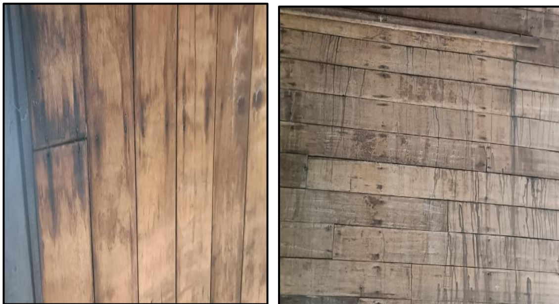
Figure 1. Leaky Wood Surfaces.
