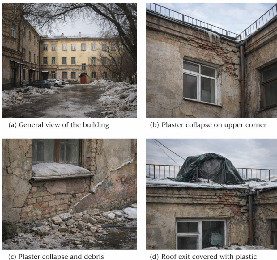
Figure 1. Multi-apartment residential building as an object of technical condition assessment of building structures.
