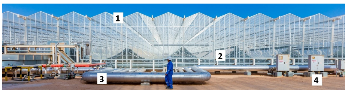
Figure 12. A front photo of the Miraah commercial project (© GlassPoint, reproduced with permission). (1) Protective greenhouse enclosure, (2) Parabolic trough collector mirror, (3) Steam distribution pipe, (4) Electrical distribution panel.
