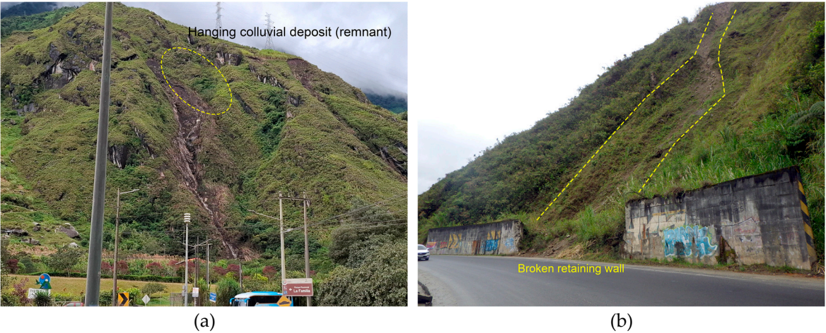
Figure 4. (a) A picture of the southern slope of the hill located NE of the Agoyán dam, showing a partially eroded surface deposit from the last rainy season in June 2024, which was channeled through the drainage system to (b) Broken retaining wall.
