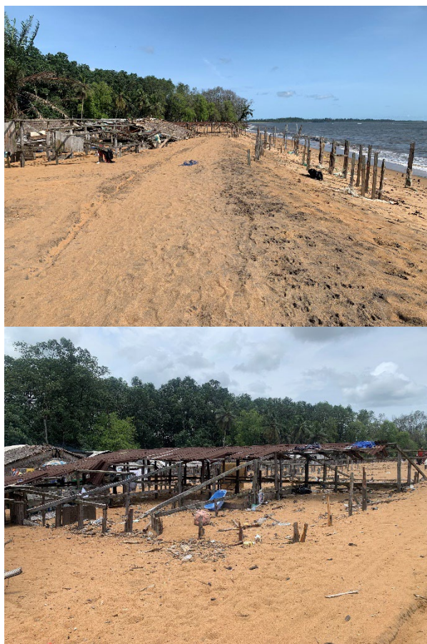
Plate 2: Homes damaged by coastal sedimentation (sand accretion) in the Douala-Edea National Park.
