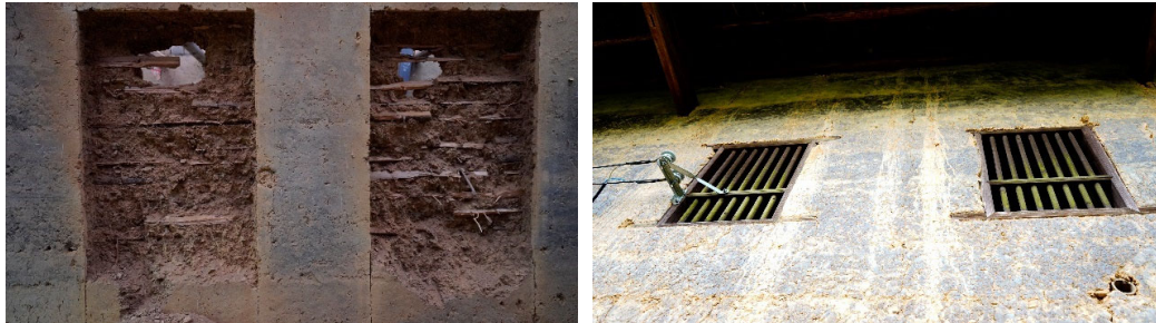
Figure 8. The internal structure of the earthen walls in the traditional rammed earth buildings of the village shows remnants of the traditional formwork and scaffolding used in construction.
