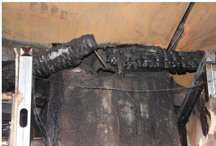
Figure 1. Image of the chimney of the fireplace structure and the ceiling of the house.
