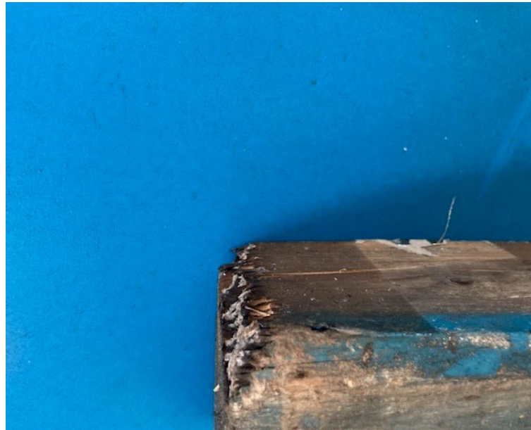
Figure 10. Image with wooden beam with evident pyrolysis and carbonization zone.
