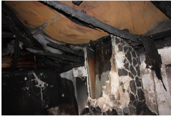
Figure 4. Place next to the fireplace where the lining, mineral wool and sandwich panel filling were completely consumed, in the living room.
