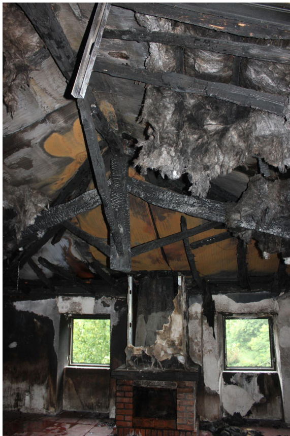
Figure 6. Spread through the living room ceiling, completely destroyed.
