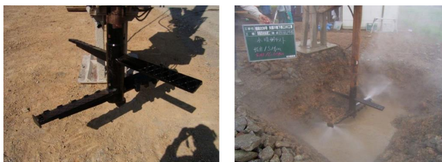
Figure 4. Water spraying demonstration by MITS monitor.
