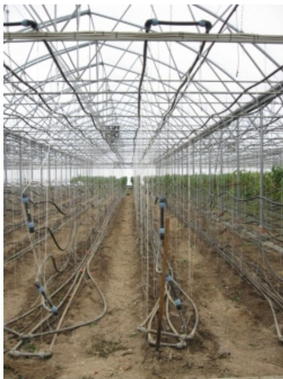
Figure 4. Heating system installed in the plant growing zone of greenhouse.
