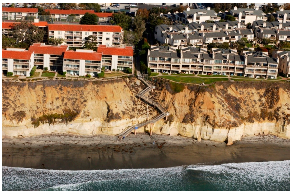
Figure 7. Eroding coastal bluff fronting the lowest marine terrace at Solana Beach, northern San Diego County (Kenneth and Gabrielle Adelman, California Coastal Records Project, Californiacoastline.org).
