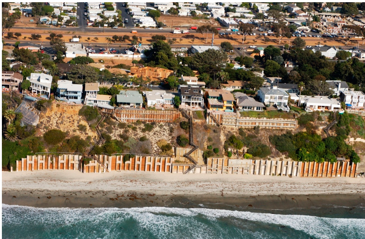
Figure 3. Continuous seawalls along the back beach in Encinitas, northern San Diego County where 34% of the entire county shoreline has been armored (Kenneth and Gabrielle Adelman, California Coastal Records Project, Californiacoastline.org).
